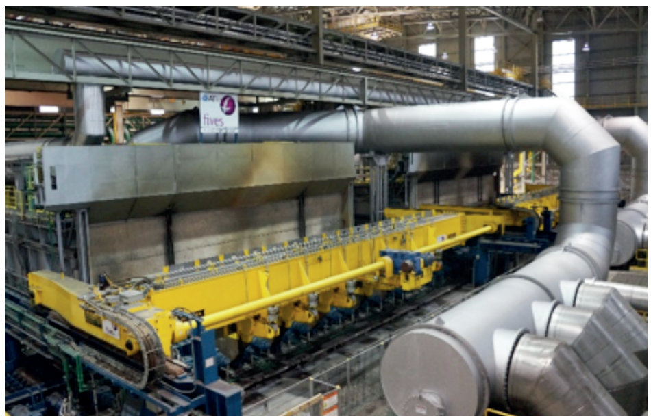
Fig 3. View over the Stein Digit@I Furnace Advanced Technology
